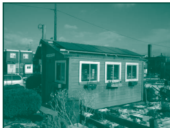
Solar panels installed on the shed at Aspen Farms
